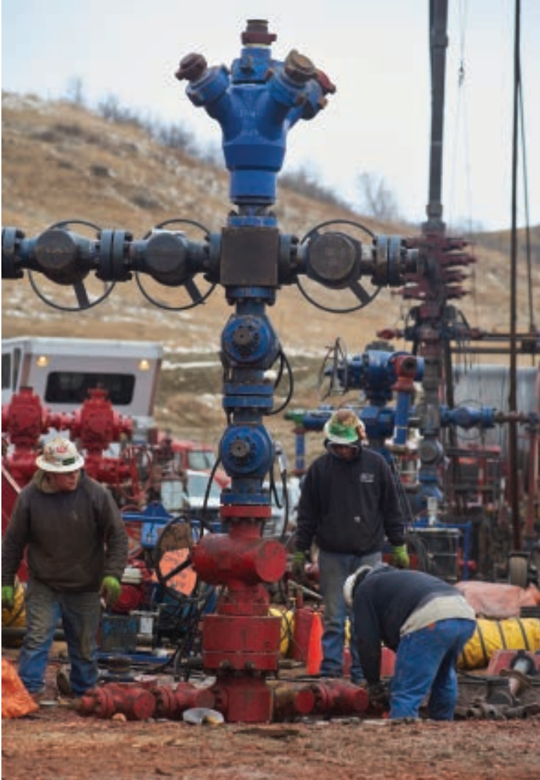
Above and at right, workers at a zipper-frack job for Whiting at a three-well pad in a hollow in Sanish Field. Discovered by Whiting in April 2006, Sanish Field produced 103 million barrels of oil through November.
