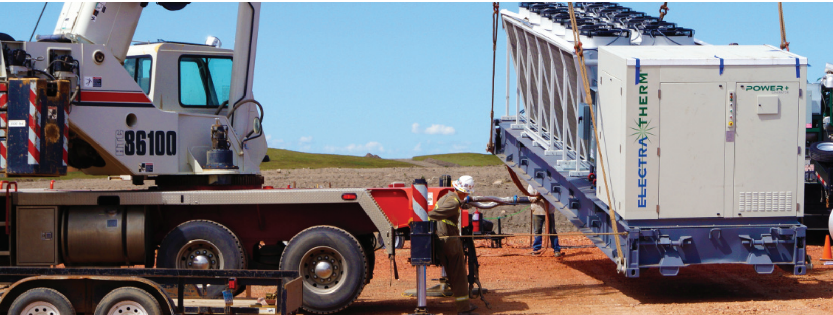
TECHNO DEMO: ElectraTherm's Power+ generator was unloaded in 90 minutes and running the same day using captured gas to produce electricity. PHOTO: ENVIRONMENTALLY FRIENDLY DRILLING
