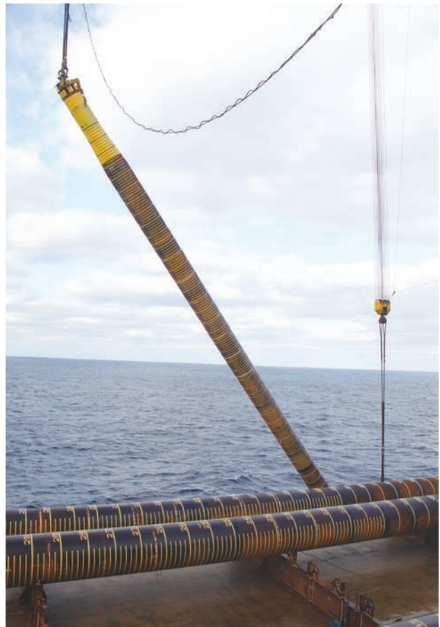
The Balder deepwater construction vessel operated by HMC lifts an anchor pile into place. (Source: Hess Corp.)
